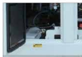
Double-layer fuel tank
