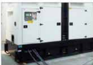
Enclosed power outlet, terminal and sockets
